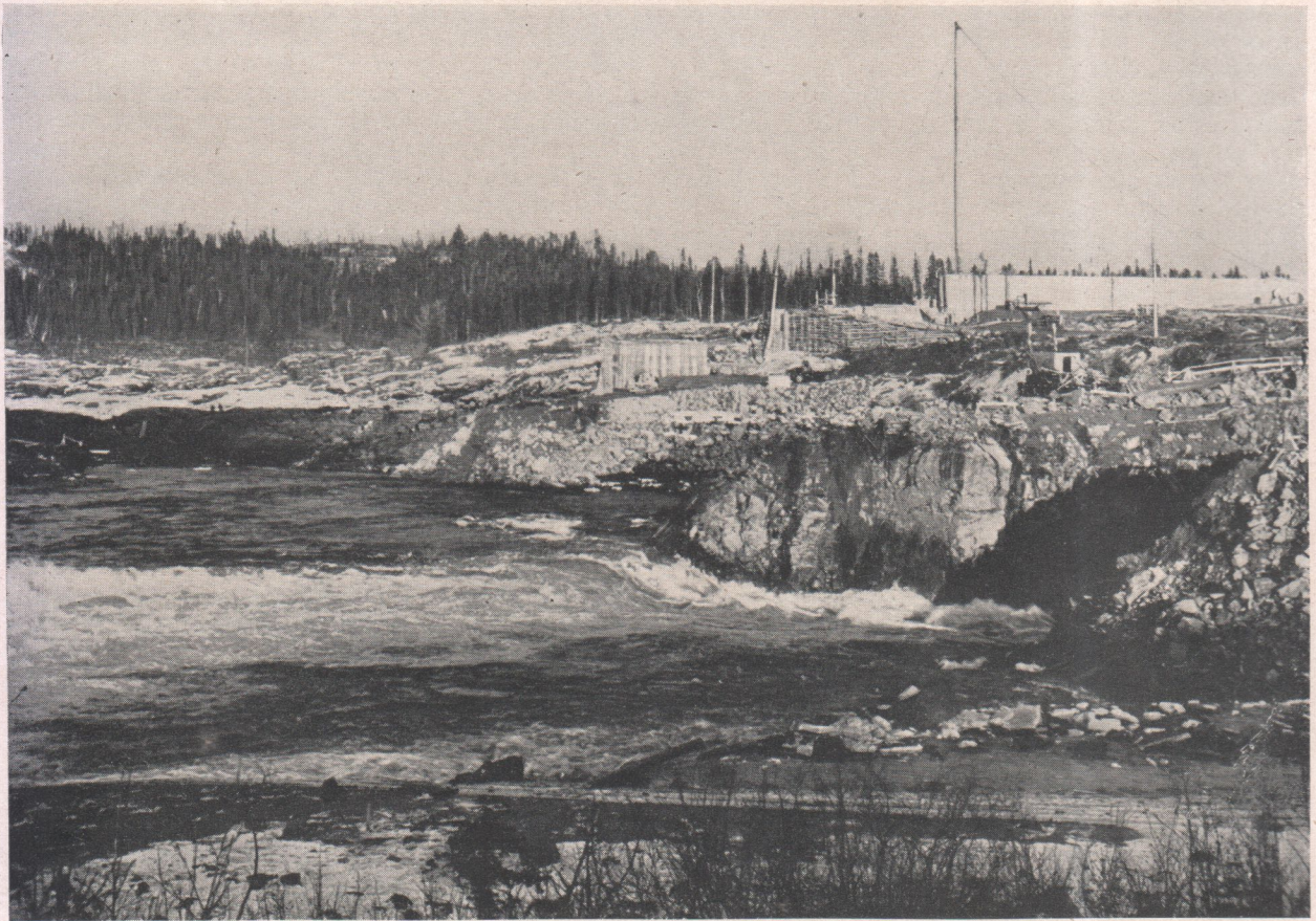
Fig. 4. The river flowing into the diversion tunnel, leaving the original bed virtually dry
