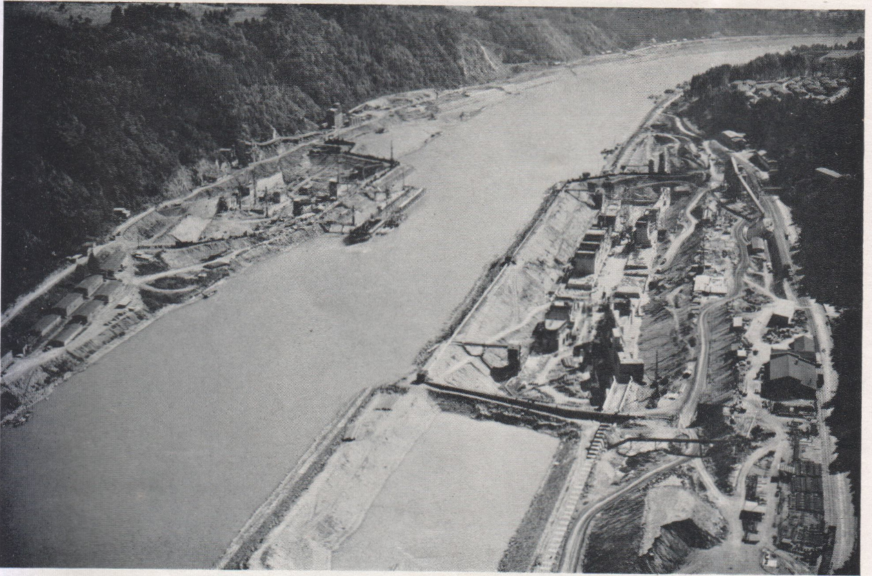
Fig. 2. Construction Section IA, looking downstream, on 30 September 1960. On the left is the construction pit for two spillway openings, and on the right the southern lock is in course of construction. The foundation pit for the upstream training wall is in the foreground
