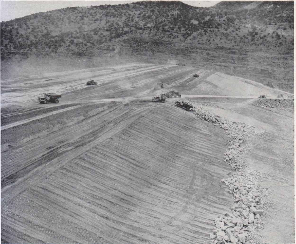
Fig. 7. Embankment construction in progress. Note the dump truck being lowered by a bulldozer to place riprap
